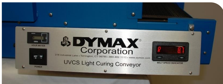
Figure 27. Conveyor Control Panel, Front
